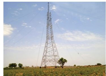
500 kV Double Circuit Quad Bundle Transmission Line from SECL Power Plant in Thar Block-I to Matiari Converter Station, Sindh
