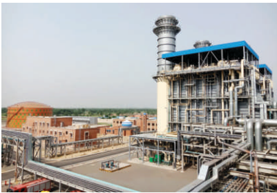
1223MW RLNG-based Combined Cycle Power Plant at Balloki, Sheikhupura
