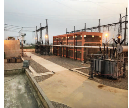
Air Insulated Switchgear Grid Station at Ghazi Road, Lahore
