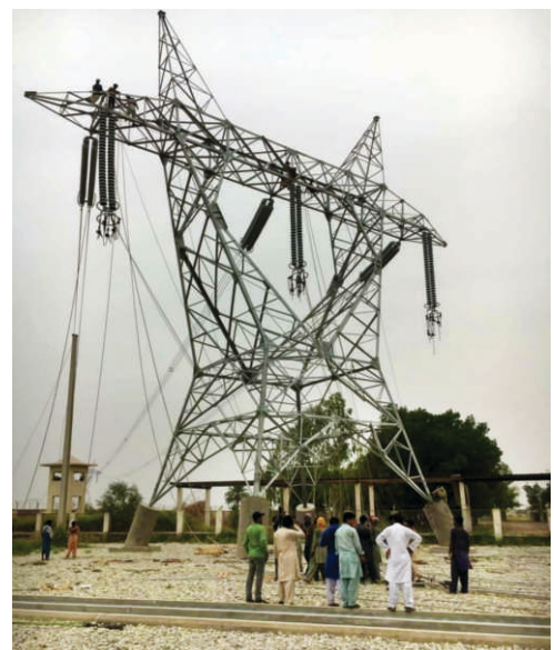
3rd Circuit Jamshoro-Moro-Dadu-Rahim Yar Khan Transmission Line and Moro Substation Project
