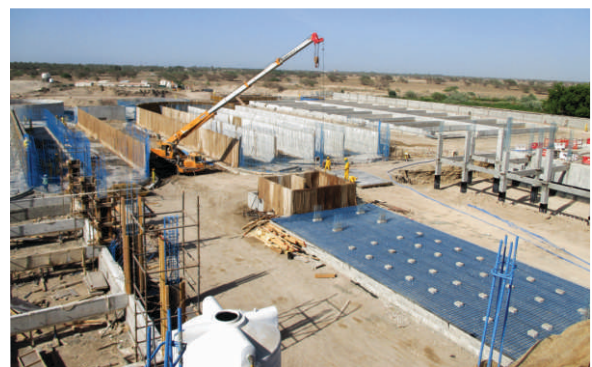
Wilayat Al-Musannah Sewage Treatment Plant, Oman
