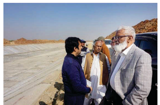
Mr. Mansoor Ali visiting the ongoing lining works on KBFU Lining Phase-1 Project, along with Mr. Imran Hussain Memon, Chief Resident, Mr. Qamar Hussain Lakhro and Muhammad Aslam Laghari
