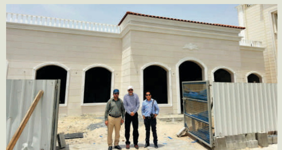
A view of addition of Majlis to existing villa at Gharaffa, Doha, Qatar
