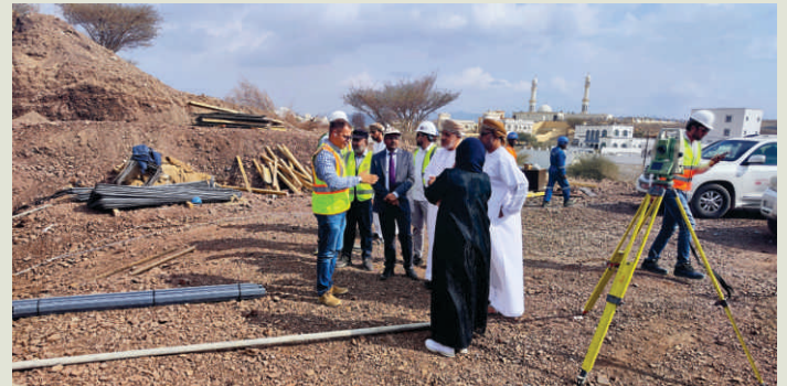
Mr. Asif Mehmood briefing the Director General, Director Design, Director Projects and Project Engineer of MTCIT, along with Engineer's Representative, NESPAK and Project Manager, Ms Galfar about the progress of work
