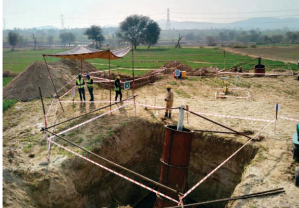
NESPAK has ensured strict adherence to the Health & Safety Measures and implementation of environmental monitoring and management plan during the execution of construction activities at site
