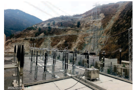
Shunt Reactors at 884 MW Suki Kinari Hydropower Project
