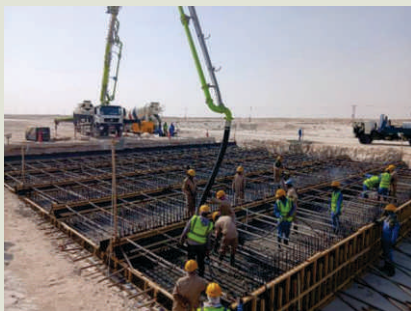
Base Slab Concrete in Progress as part of the Sultan Said Bin Taimur Road Project
